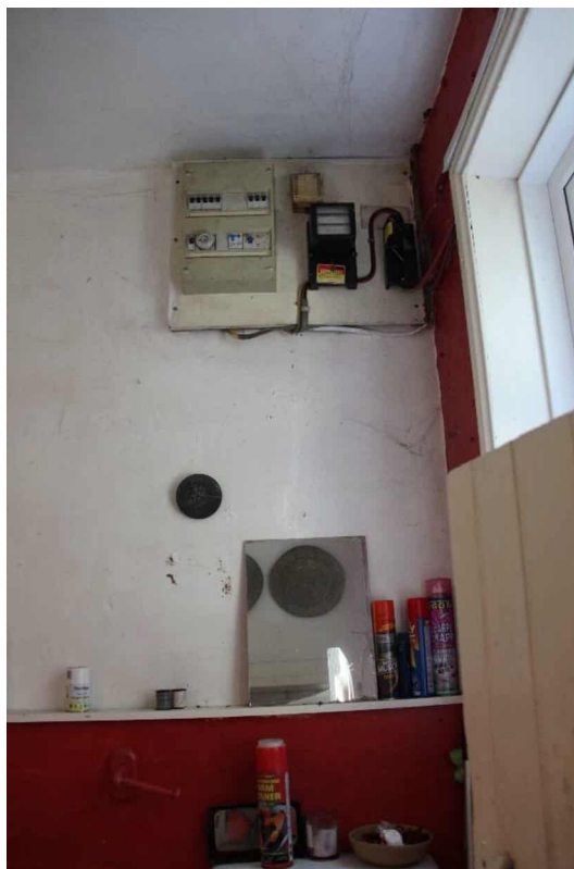
Photograph 43 - View of fuse box and meter
