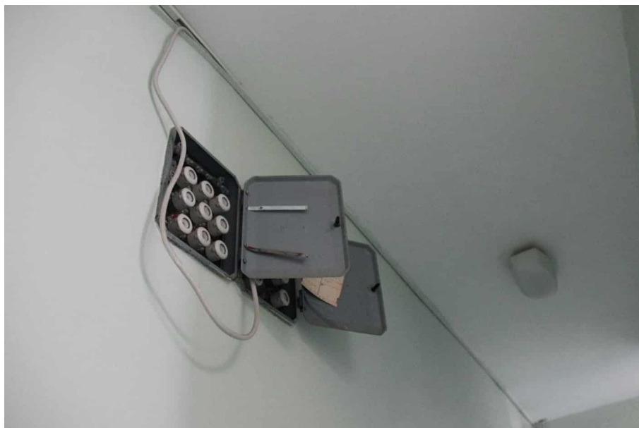
Photograph 58 - Fuse box on 2nd floor.
